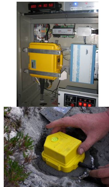
Fig. 4. Up: Data acquisition system of geophone network installed in the upper bunker. Down: Installation of a 3-component geophone.
