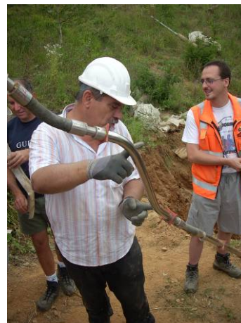
Fig. 10. The deformed module of D.M.S. column showing the displacement of about 60 cm.
