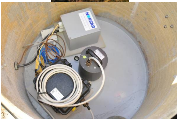
Fig.5. Up: Installation of the broadband seismic station AKN. Down: Seismometer pit with sensor, power/communication module and data acquisition module.
