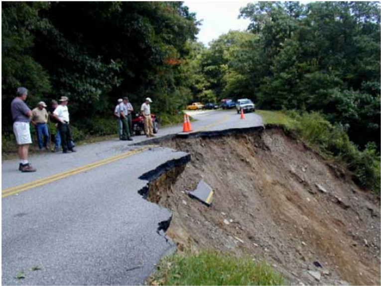
Figure 4.6.4 Example of road fill in North Carolina (USA) that initiated a debris-flow. This occurred during heavy rainfall (From Collins, 2008).
